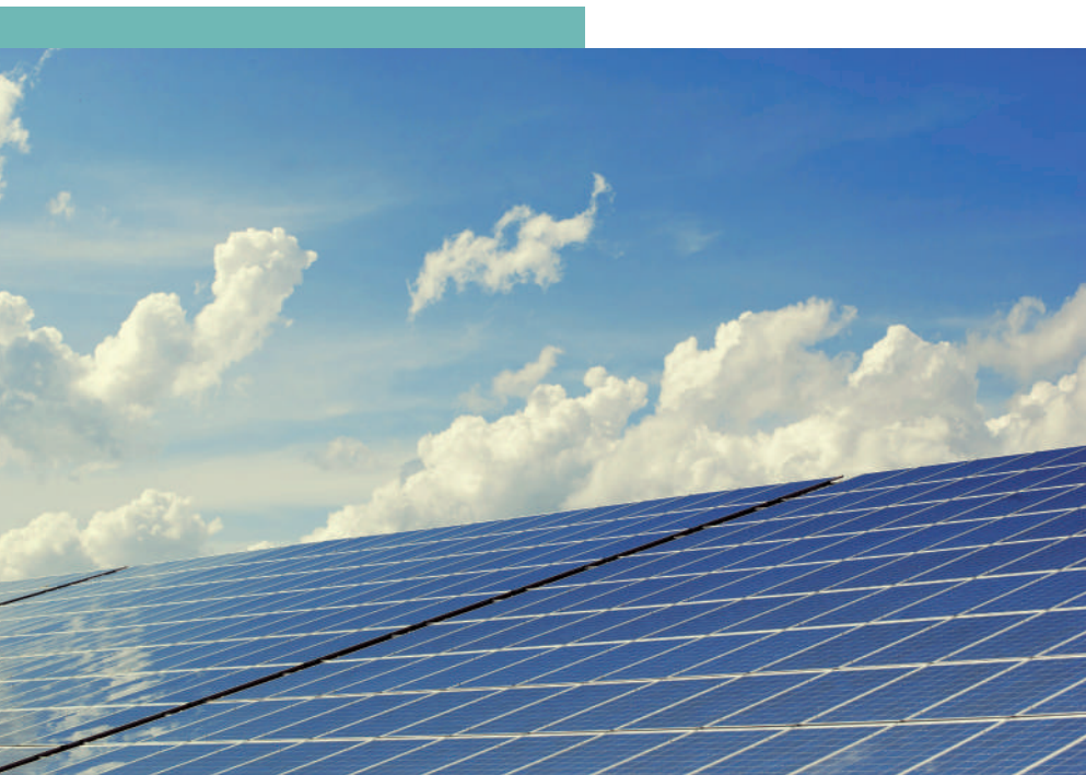
Figure 4.2. Photovoltaic panel. Source: Pixabay.
